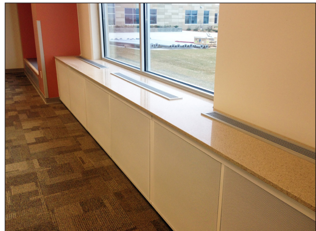
Multiple TAO units installed in an elementary school
