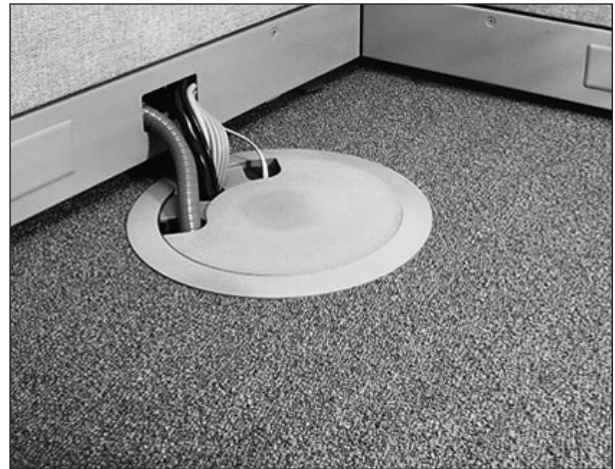
TAF-G diffuser installed in a cubicle
