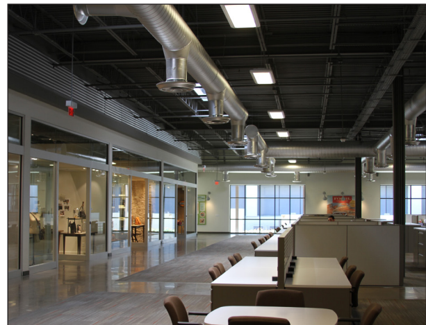
TMRA-AA installed in an office environment
